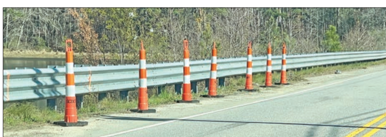
Orange cones mark areas along the road where erosion of the dam is inching toward the roadway.
