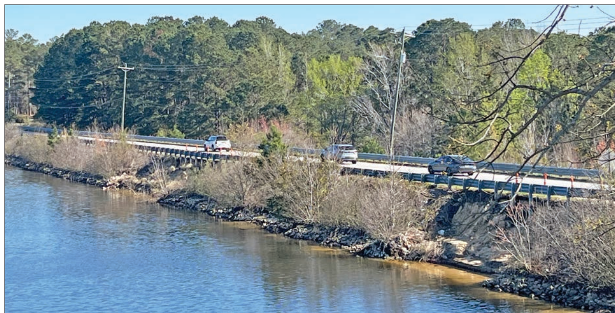
This view of Longtown Road West over the Lake Columbia dam shows two large erosions on the dam.
